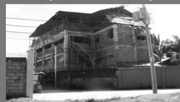
Here is the dorm as of Dec 2007. Tarp and tin covers the windows 2 prevent wind/rain damage.
