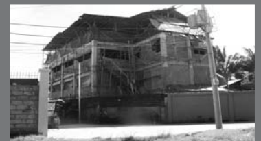
Here is the dorm as of Dec 2007. Tarp and tin covers the windows 2 prevent wind/rain damage.
